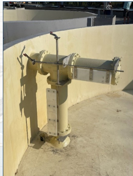
PHOTO 4: Flow control baffles to control angular velocity on inlet feed water piping
