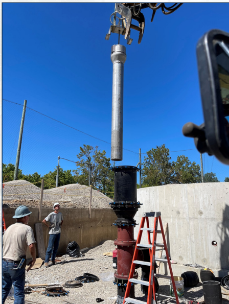
PHOTO 3: Installation of telescoping valves to regulate underflow
