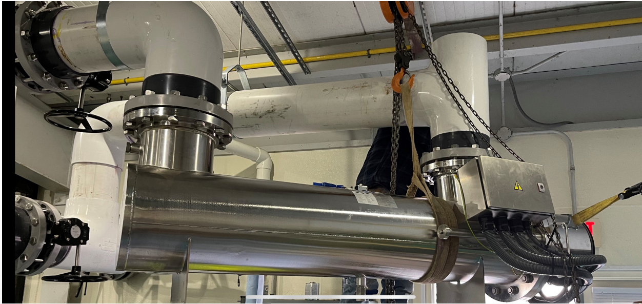
PHOTO 6: Picture of the new 260 gpm UV disinfection unit to eradicate IPNV
